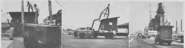
LAGO TOOL shed heads for Oranjestad site where it will be utilized by Philipsena Girl CUARTO DI warda berment di Lago ta bai pa Oranjestad na un sitio na banda di lo words. Girls will use shed as a store room for the time being. Later on the building will be part of an extension project.
